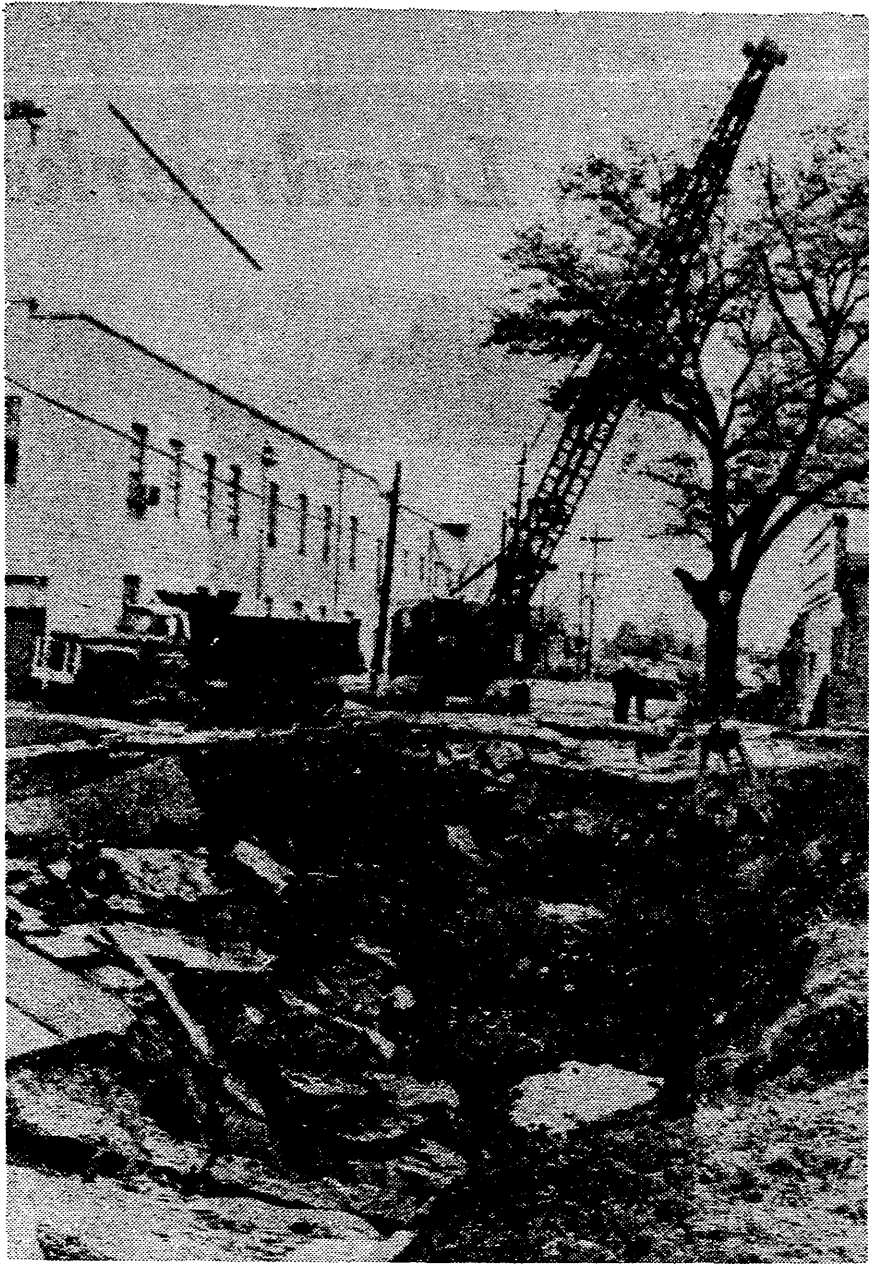
$200,000 POTHOLE — Work has begun at the site of a street cave-in on Calypso St. in Monroe. The cave-in began as a sagging spot in the pavement, and Monday the street fell in. The city council declared a state of emergency and began
